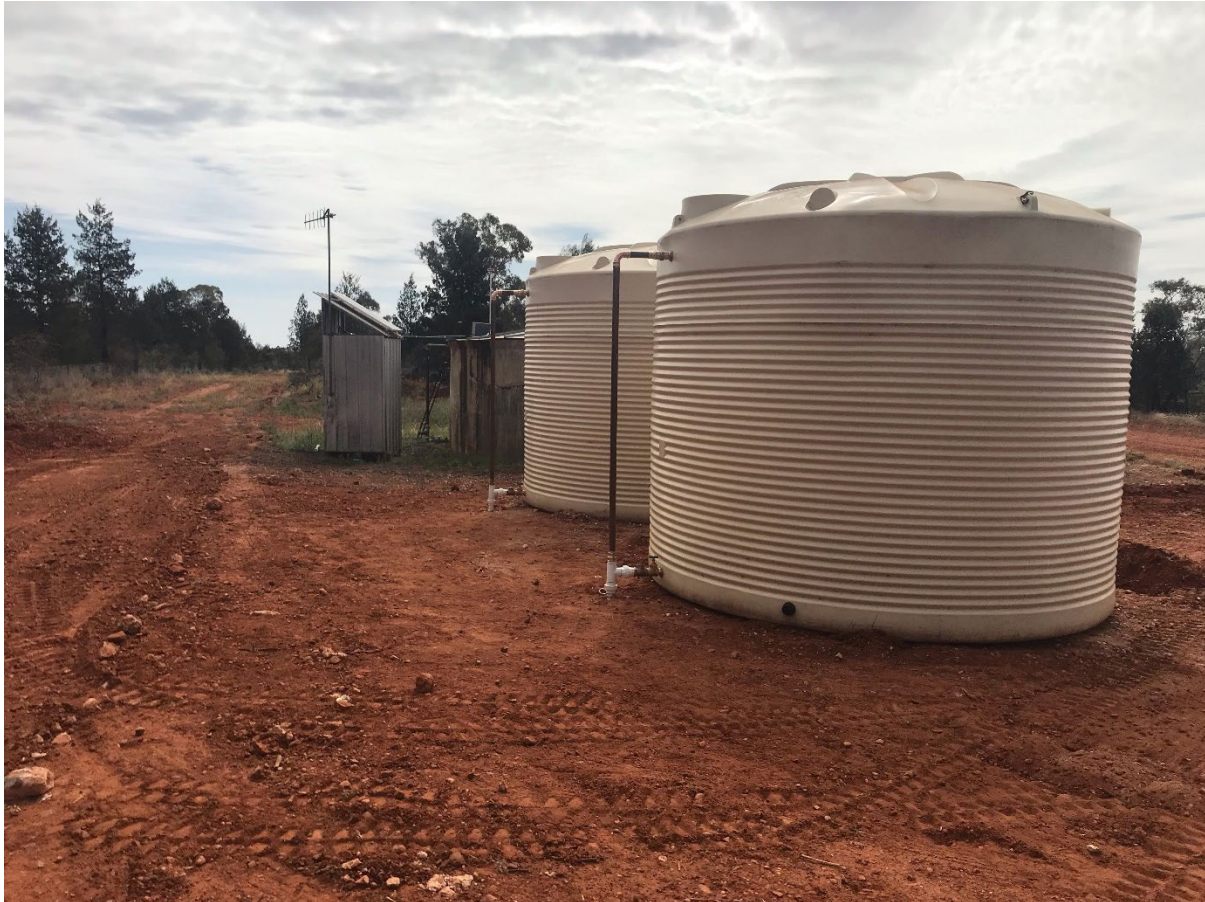
Photo: Additional water storage tanks at Y4 on Holden Road (Yoolaroi water scheme)
