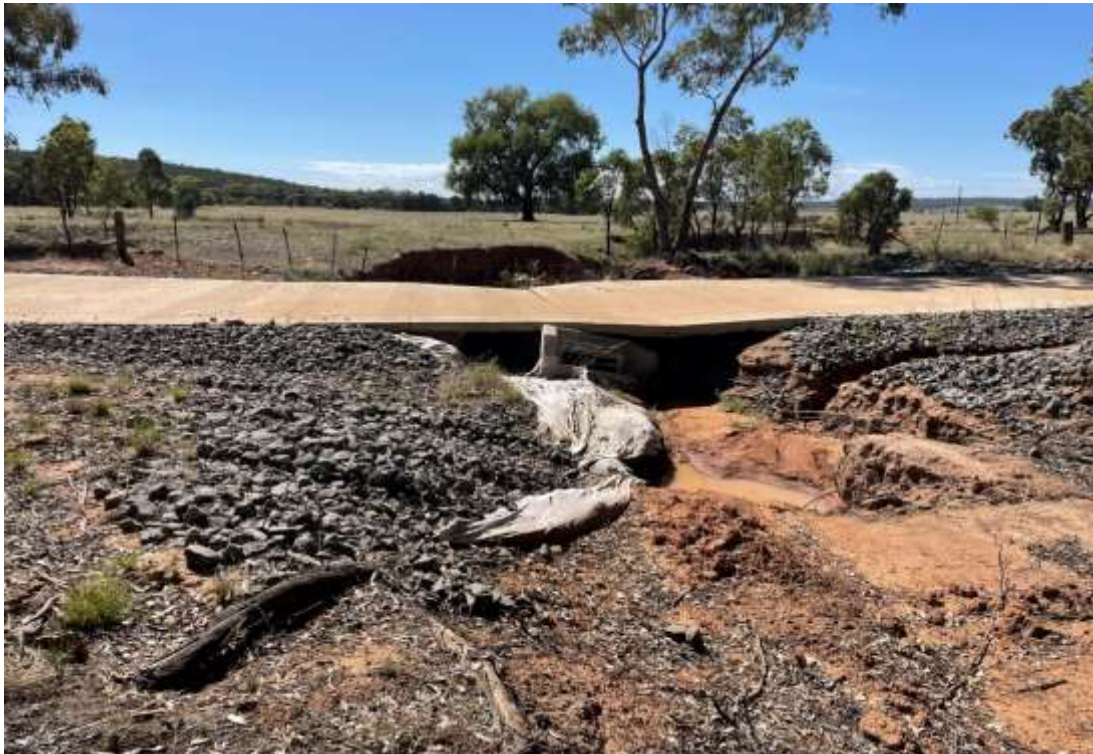
Cannards Road; Causeway, upstream view, undermined by flooding.
