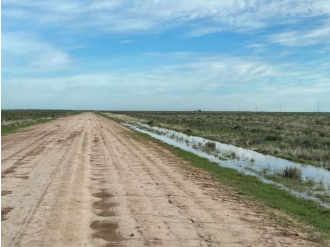
Photo 2: Lowlands Road. Minor rivulets can be seen where the water has moved from the road pavement towards the table drains. The road has a cross fall of 3% from the centre line of the pavement.
