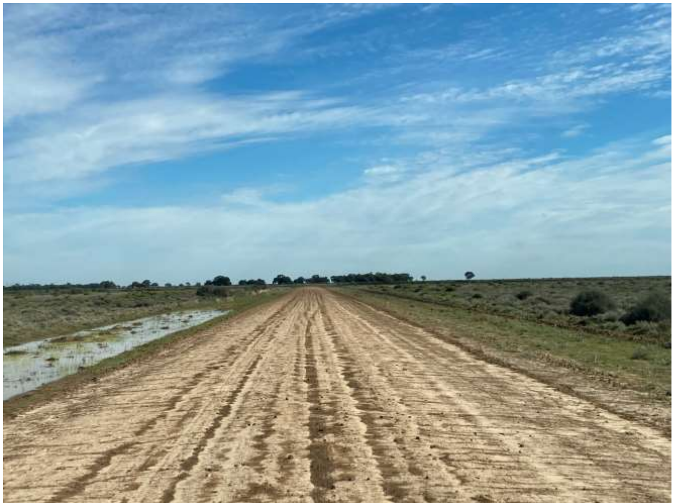
Photo 1: Lowlands Road. The road pavement has a high clay constituent which becomes extremely adhesive and slippery when minimal rainfall has taken place. The photo indicates the water run off into the table drains from the pavement which shows no signs of water ponding leading to potholes and other pavement defects.
