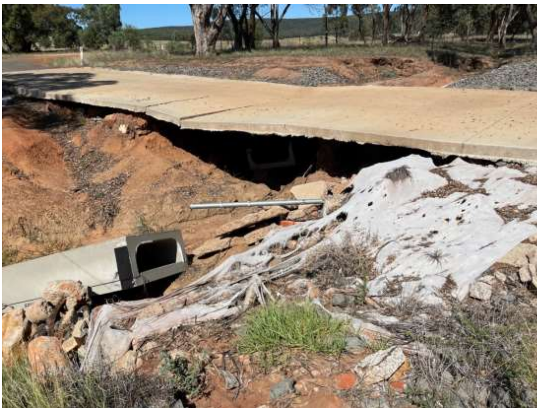
Culverts washed out downstream, detour was set in place to maintain traffic flow.
