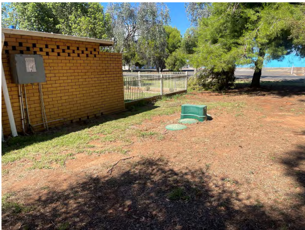
Photograph 23: Septic system for public toilets. Photograph taken facing west.
