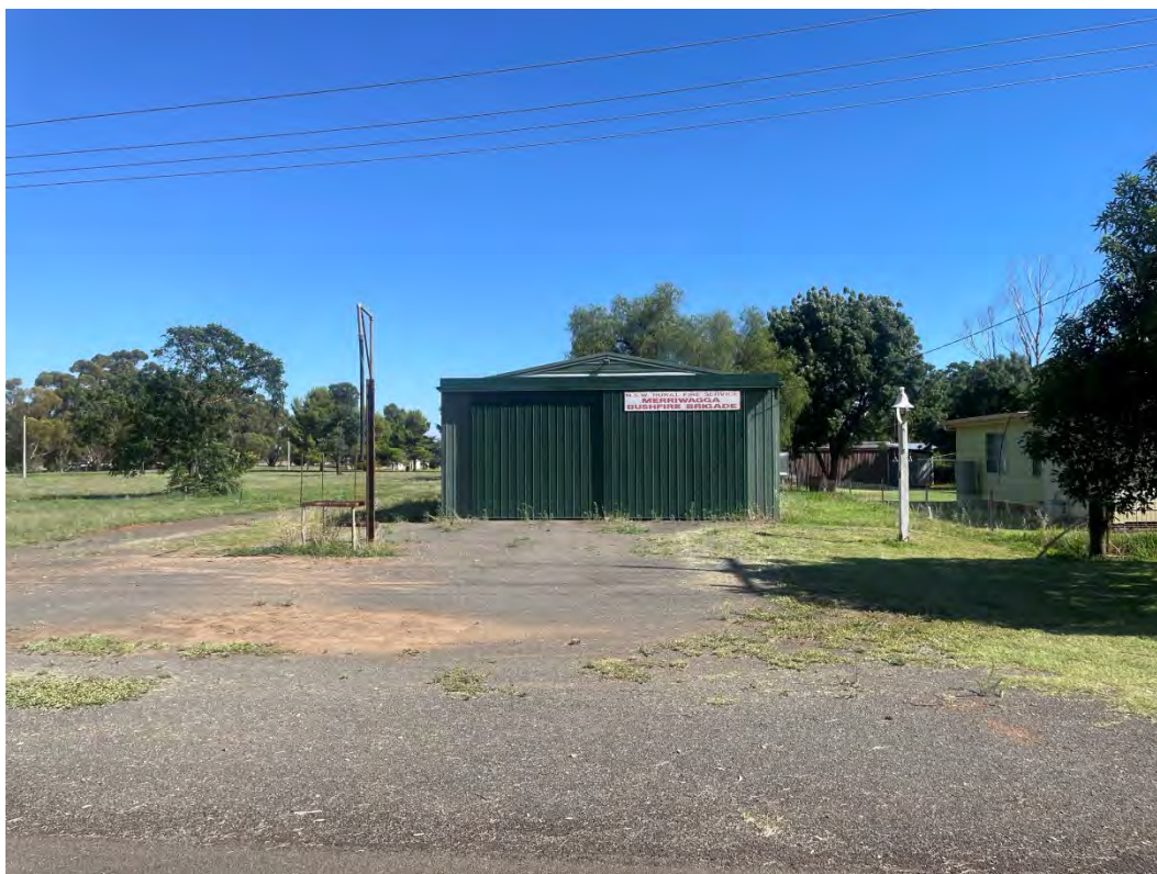
Photograph 19: Steel shed on grade slab for the NSW Rural Fire Service Merriwagga Bushfire Brigade. Photograph taken facing north.
