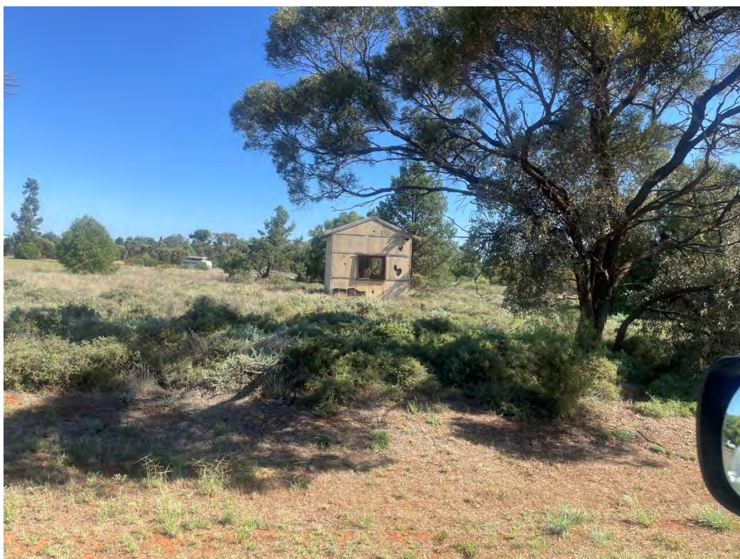
Photograph 20: Shed clad with ACM in the north of the site. Photograph taken facing north.
